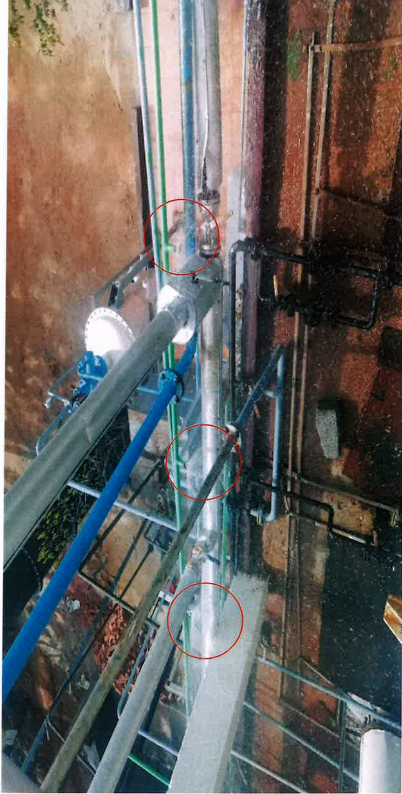
Provided odour suppressant mist spray/sprinkle PIIAN liquid system at ZLD and ETP area to control VOC's.
